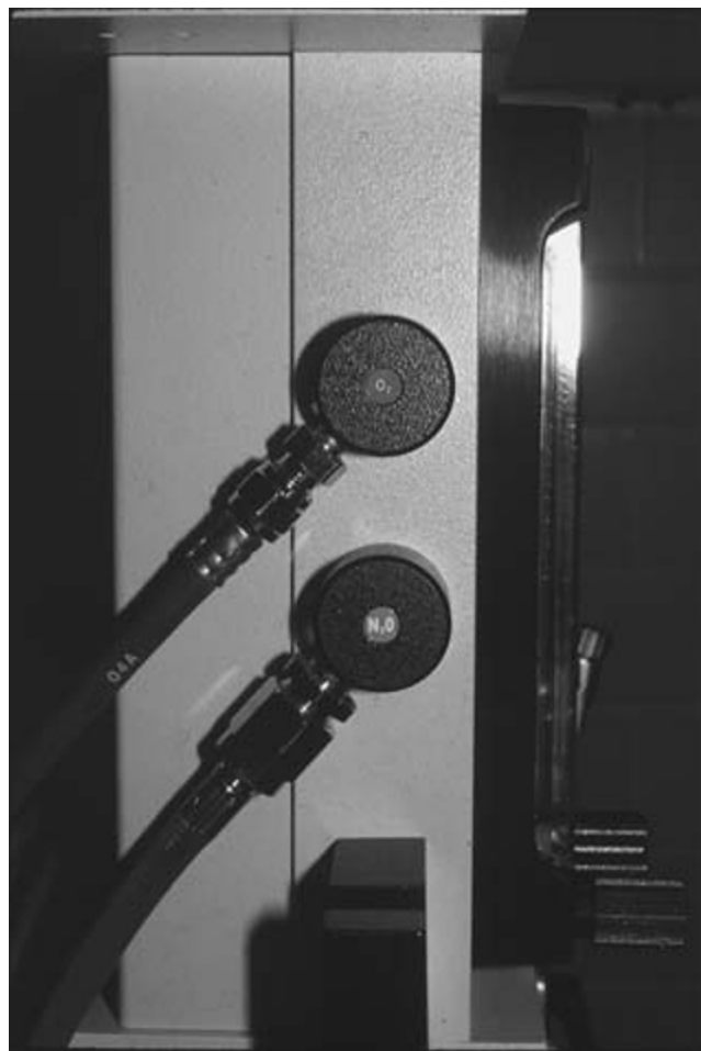
Fig. 17.5. Pipeline inlets for oxygen ( top connector labeled as O 2 ) and nitrous oxide ( bottom larger connector) on a Drager anesthesia machine (North American Drager, Telford, PA). The female diameter index safety system (diss) connectors from the high-pressure hoses couple to the male diss pipeline inlets on the anesthesia machine.
