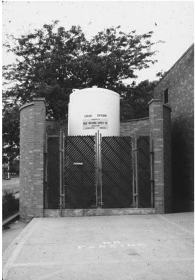
Fig. 17.2. An outside bulk container for liquid oxygen supplying the central medical gas pipeline system of a large hospital.
