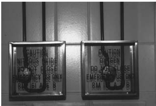
Fig. 17.3. A set of emergency shutoff valves for oxygen and nitrous oxide in a central pipeline system for medical gases in a veterinary teaching hospital. These valves should be placed strategically throughout the gas distribution system to control the flow of gases during emergencies or maintenance.
