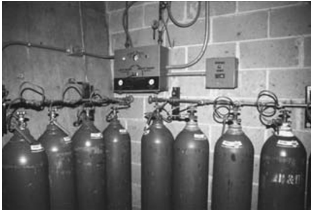
Fig. 17.1. Primary and reserve banks of large oxygen cylinders supplying the central medical gas pipeline system at a veterinary teaching hospital. The primary bank supplies oxygen to the pipeline system until the cylinders are depleted, at which time the system is automatically switched to the reserve bank.
